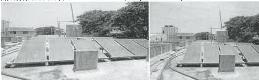
SOLAR WATER HEATER PANEL IN HOSPITAL
